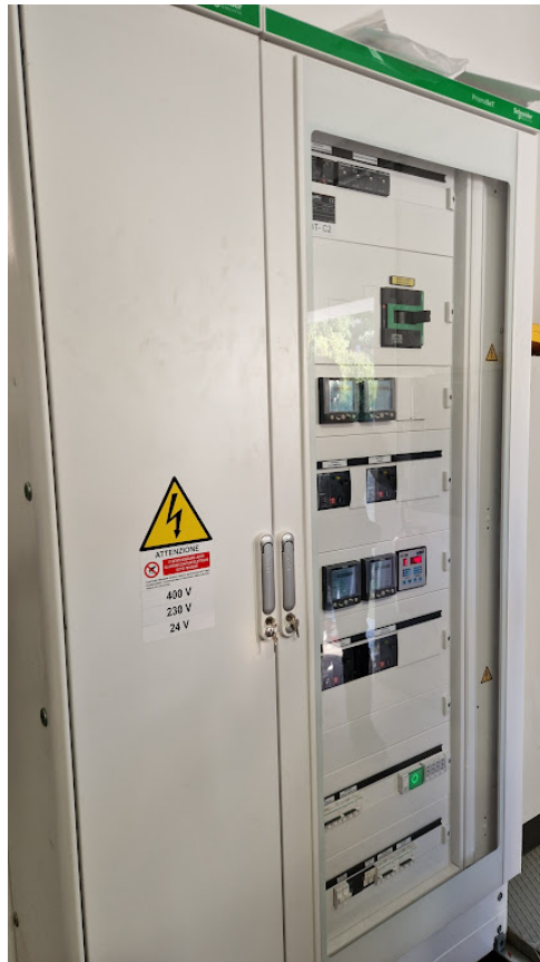
Figure 5.1: Berchidda Low-voltage distribution panel inside an electrical substation, an example of an asset being monitored for Digital Twin implementation.
