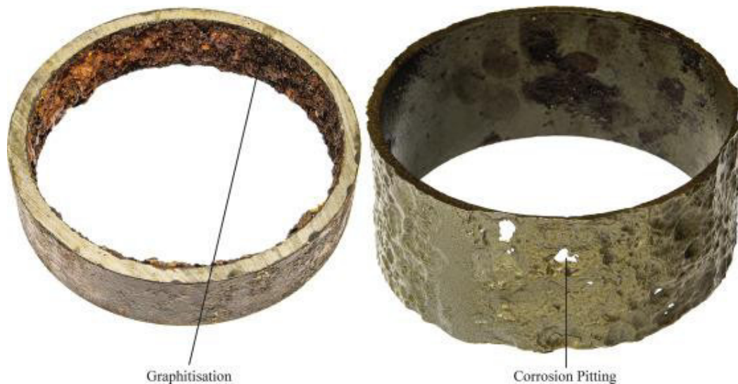
Figure 15. Reproduced from Barton et al. (2019) [40]. Examples of corrosion and chemical degradation observed in cast iron pipes. The image shows two typical deterioration phenomena: graphitization (left), in which the metal matrix is progressively replaced by residual graphite, and pitting corrosion (right), characterized by the formation of localized cavities that weaken the wall of the pipe to the point of perforation.
