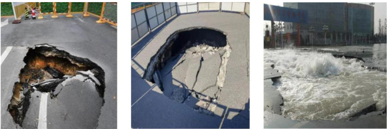
Figure 5. Reproduced from Liu et al. (2024) [16]. Typical road collapses due to leaking underground pipes in China: left, seepage from a drainage pipe; center, water leaking from a rainwater pipe; right, rupture of a pressurized water pipe (image by Yi-Chun Cao).
