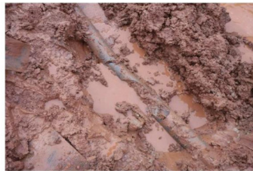
Longitudinal split on a polyvinyl chloride pipe.
