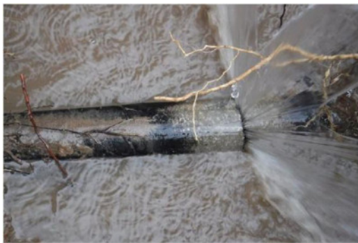
Circumferential break on an asbestos cement pipe.
