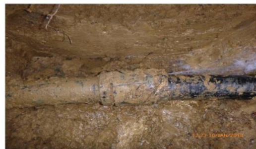
Joint failure (disconnection or gasket failure) on an asbestos cement pipe.
